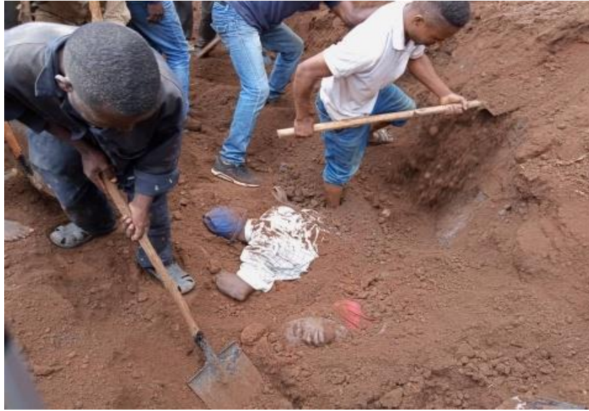
Figure 5: Soil collapse in Goma – picture taken by Cooperative Miniere BUUMA-COMIBU agent in 2019
